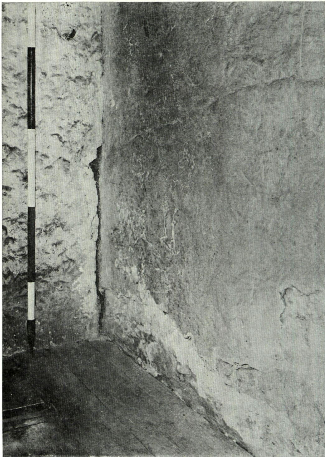
Plate 5. Titchfield Church, north-west angle of upper stage of tower, showing how the north wall of the tower (left) was built up against the west wall of the nave with a straight joint. The plaster on the west wall of the nave can be seen to pass behind the joint. (Photo. M. Biddle, Winchester Research Unit.)
